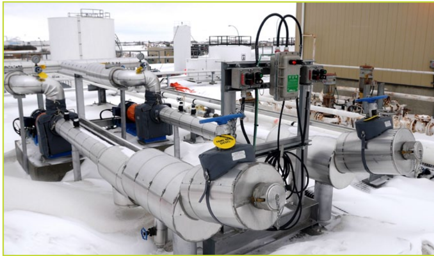
FIGURE 10: Insulated and Heat-Traced Offloading Station
