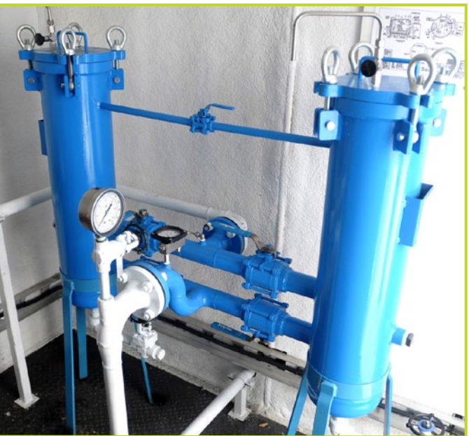
FIGURE 9: Filters on Neat Renewable Diesel Tanks
