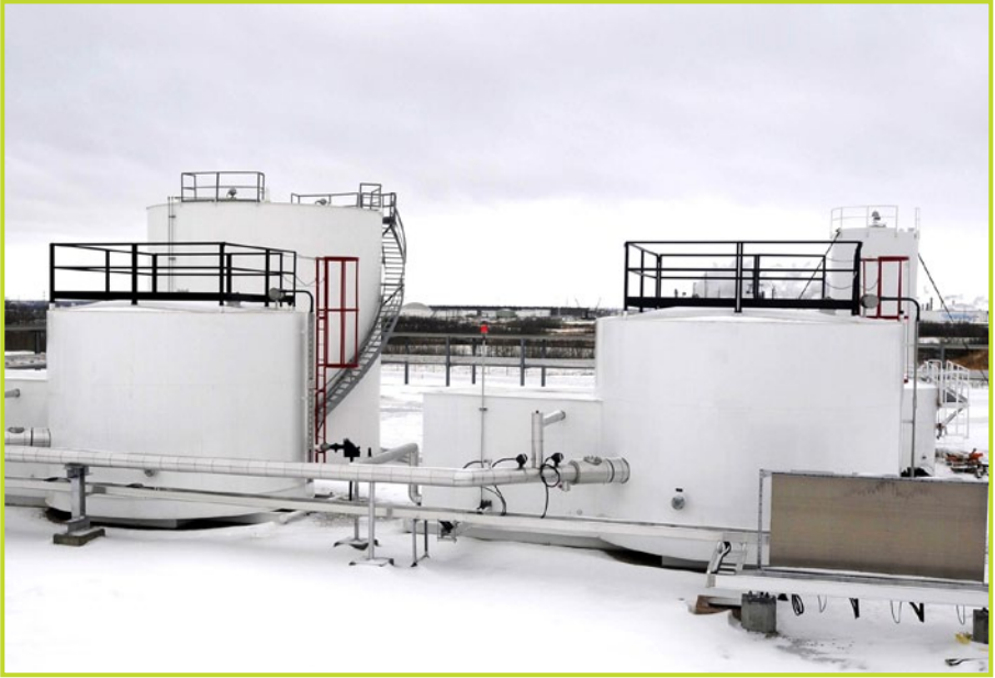
FIGURE 8: Storage Tanks for Neat Renewable
